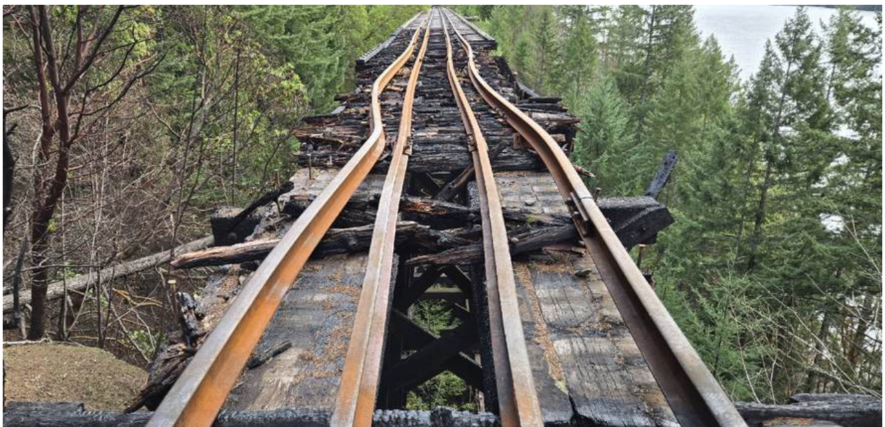
Bridge damage due to Wesley Ridge wildfire
